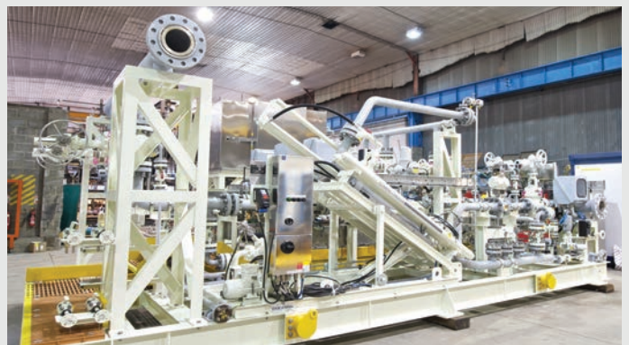
Nexen Petroleum Golden Eagle Oil & Gas Metering (UK Offshore)
