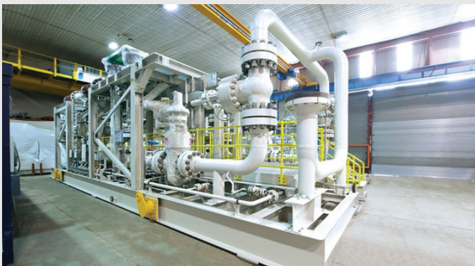
BP Clair Ridge Metering Package (UK Offshore)
